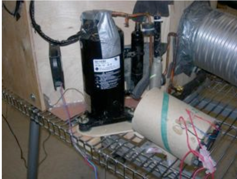
Figure 187: Extra cooling fans added to cool the compressor
