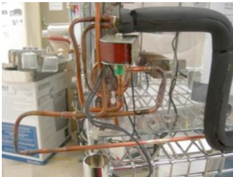
Figure 180: The extra pipes soldered to the condenser
