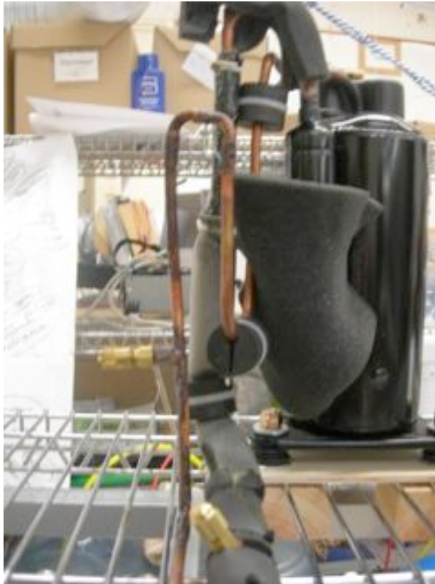
Figure 181: The extra pipes connected to the condenser with valves to add/reduce the amount of refrigerant
