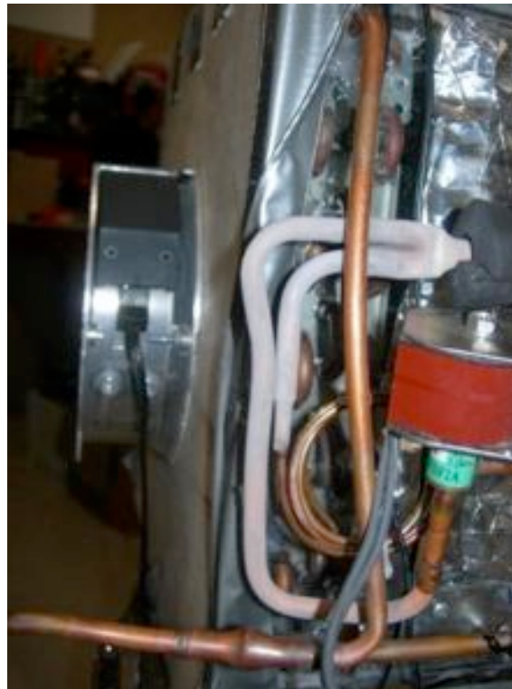
Figure 184: The frost that formed on the evaporator coils on running the prototype
