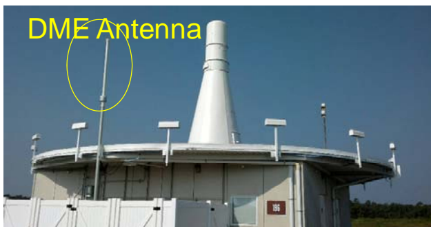
Figure 4. FAA Technical Center Test VOR TACAN (VORTAC) Station with DME monitor antenna highlighted
