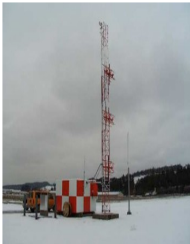
Fig. 2. Glide Slope Antenna
