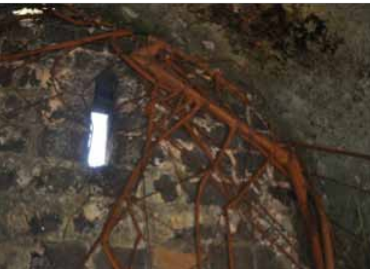
Roof collapsing due to the growth of vegetation and roots © AGTF
