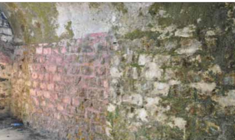
Fungal development on the walls of the barracks © AGTF
